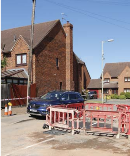
Burst water main Wednesday, traffic flowing Friday. In Praise Of Page 7
